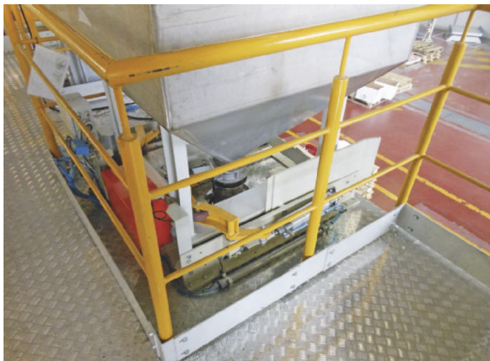
The bagging section of the line comprises fully automatic valve bag fillers
